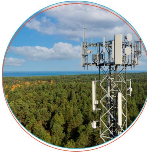
PtMP base station backhaul
